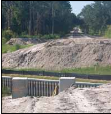
Looking toward WH at the site of the to-be-constructed bridge over the Hartridge-Conine Canal
